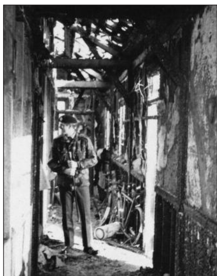
WO2 Pete Markley, SSM 13 Squadron, examines the charred remains of the squadron office – a sad end to a building known to so many.
