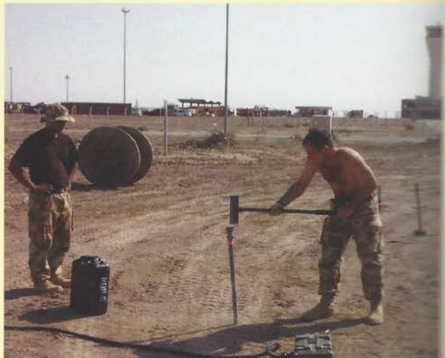
Earthing the generator - one of the mundane tasks during field deployment
